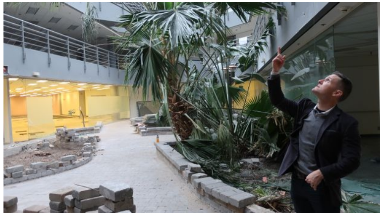
Jon Dorman, Bluebird's managing director for global development, surveys the lobby of the former National Post building in Toronto's Don Mills suburb. The building is being renovated into a three-storey storage facility.
