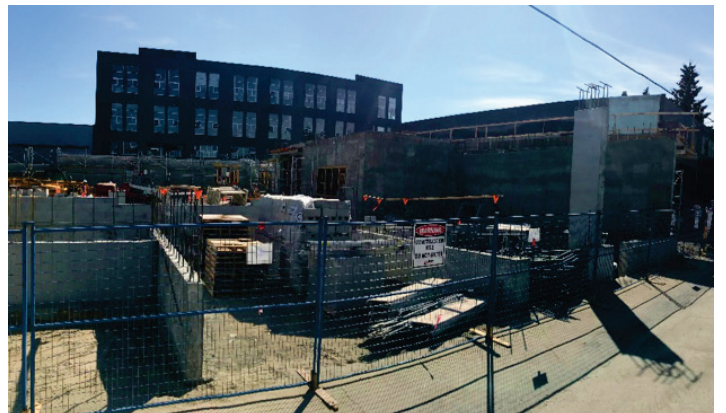
The first of the exterior walls erected on the Pender Property, August 2018
